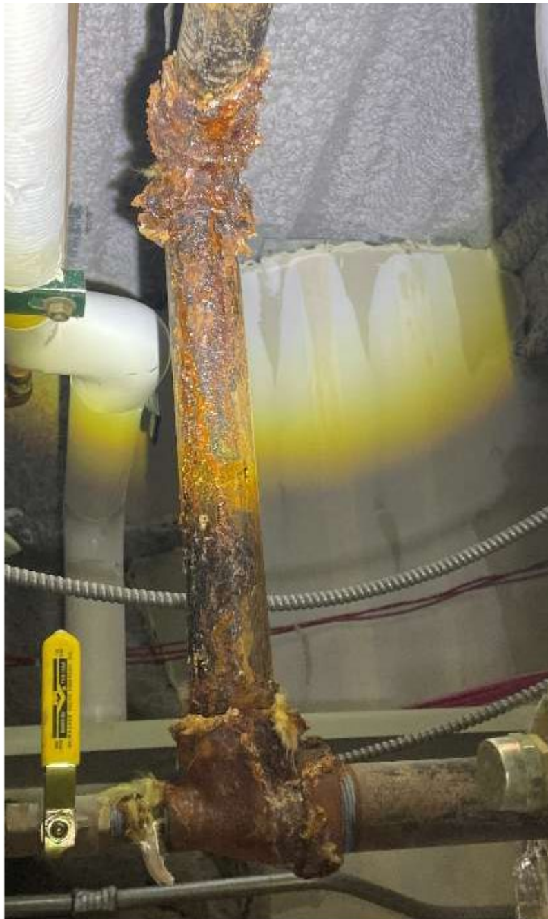
Example of Corroded Heat Piping Condition
