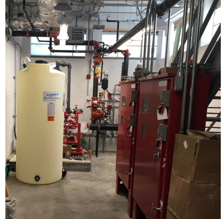
Existing foam fire suppression system
