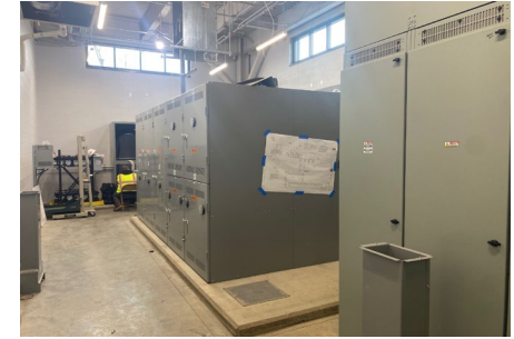
Interior Electrical Gear
