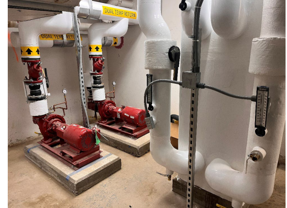
Rogers Hall Dual Temperature Pumps & Heat Exchanger
