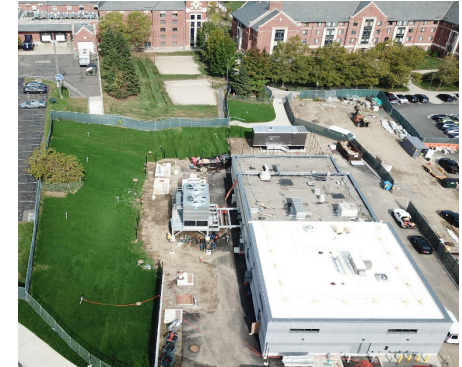
South Campus Chiller Plant Addition
