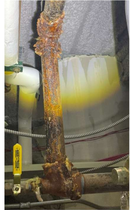
Corroded heating pipe
