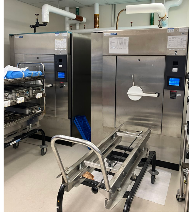
Existing sterilizer equipment
