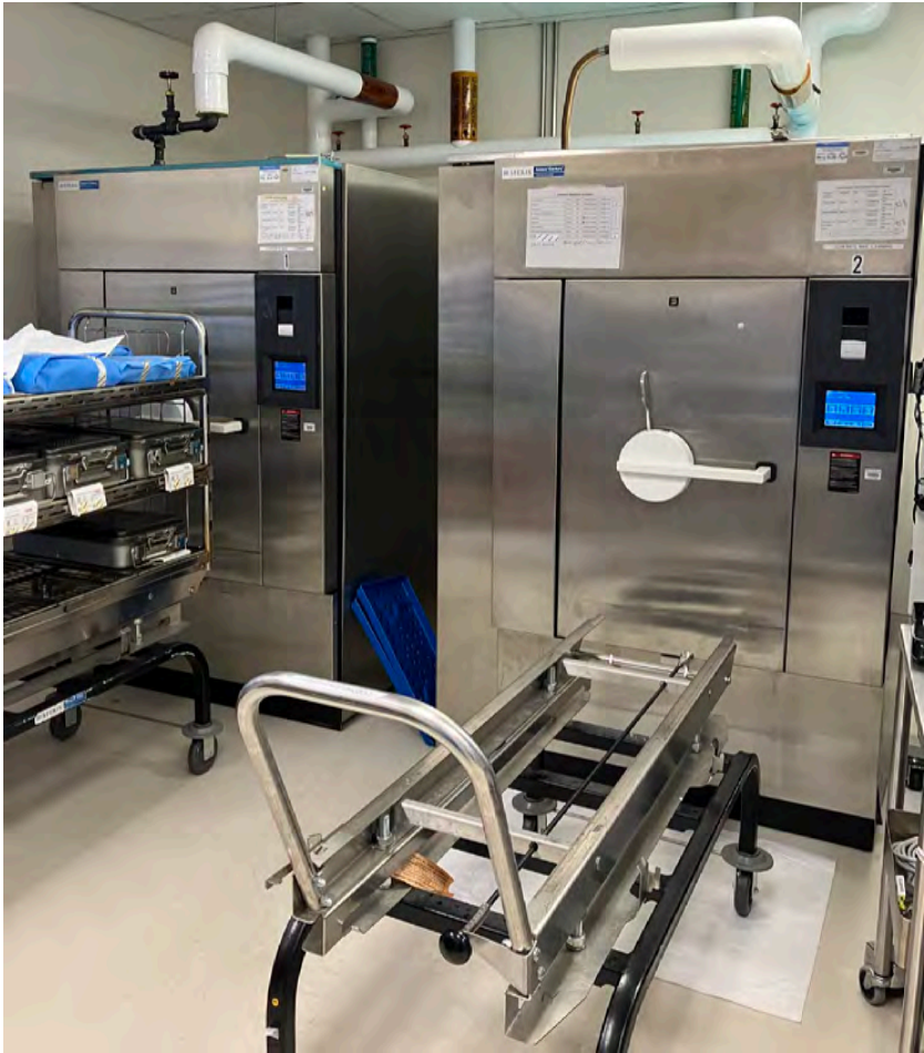
Existing Sterilizer Equipment
