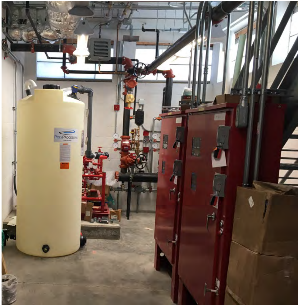
Existing Foam Fire Suppression System
