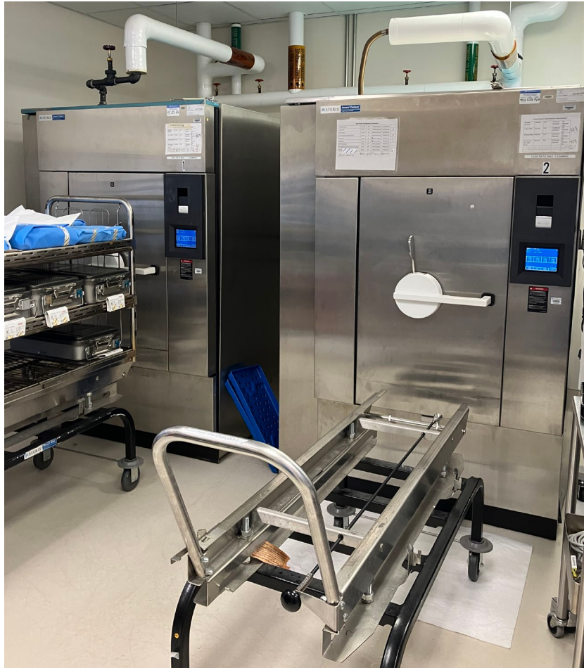
Existing Sterilizer Equipment
