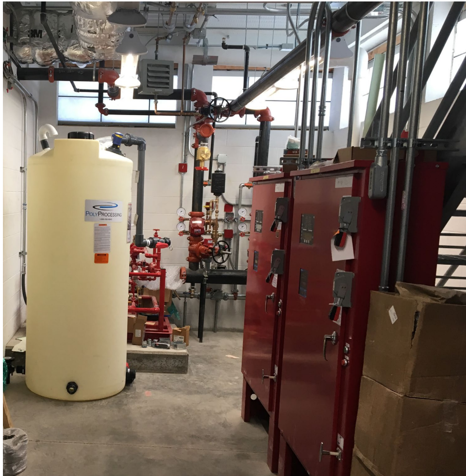
Existing Foam Fire Suppression System
