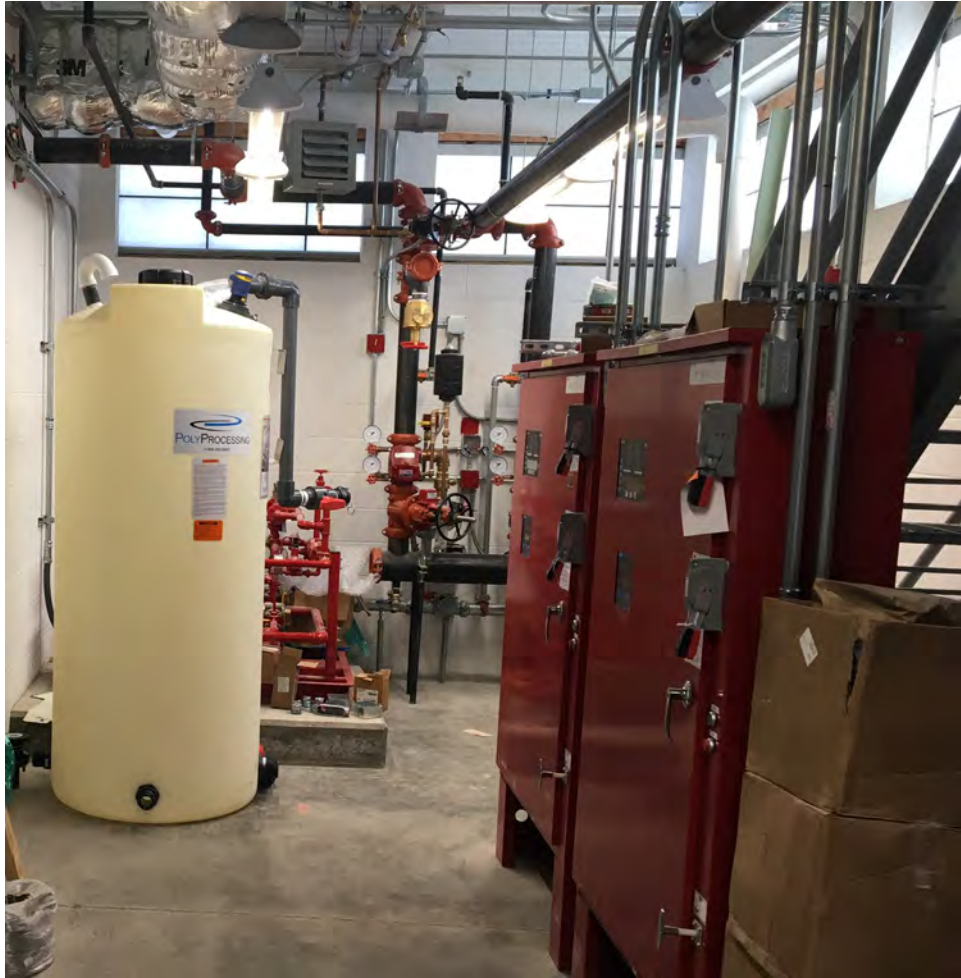
Existing Foam Fire Suppression System
