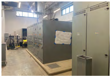
Interior Electrical Gear
