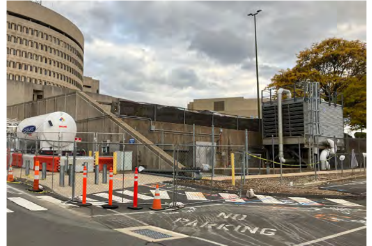
View of temporary oxygen tank unit and location of new tanks
