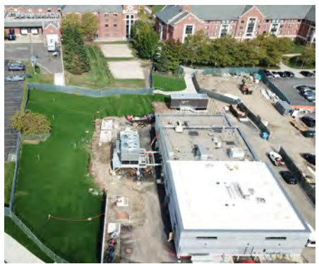
South Campus Chiller Plant Addition
