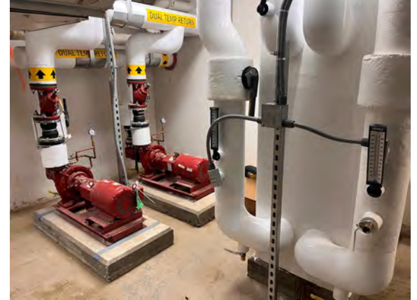
Rogers Hall Dual Temperature Pumps & Heat Exchanger
