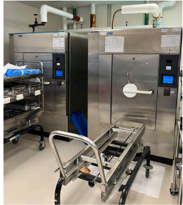
Existing sterilizer equipment
