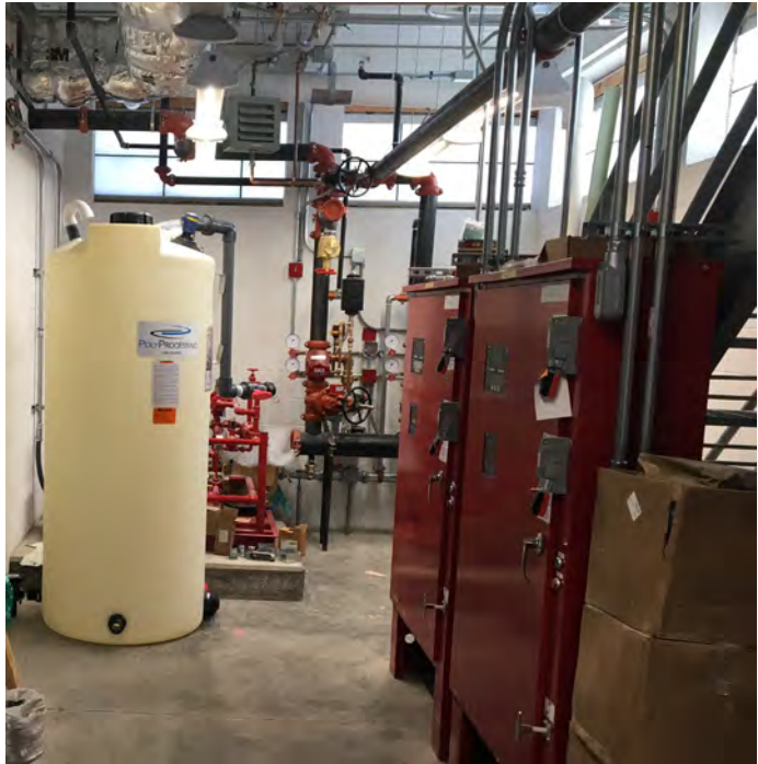
Existing foam fire suppression system
