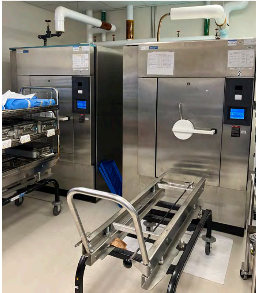
Existing Sterilizer Equipment
