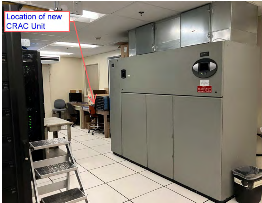
Location of New Data Center CRAC Unit
