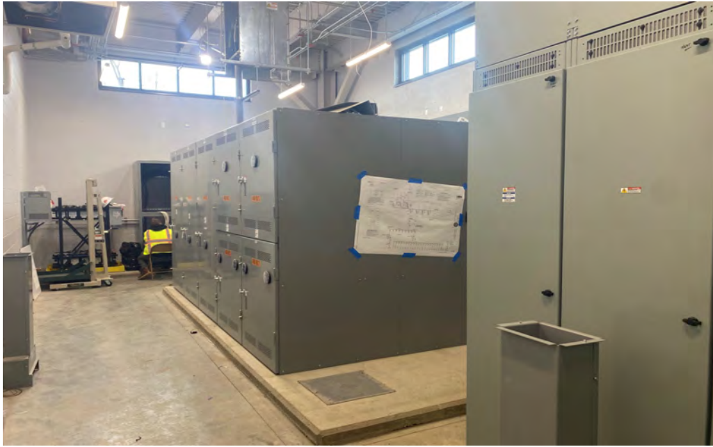
Interior electrical gear
