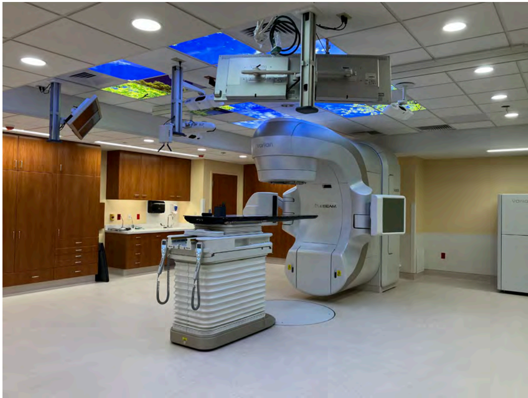
S1868 New LINAC unit
