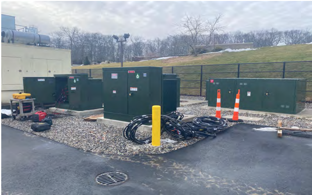
Exterior electrical gear
