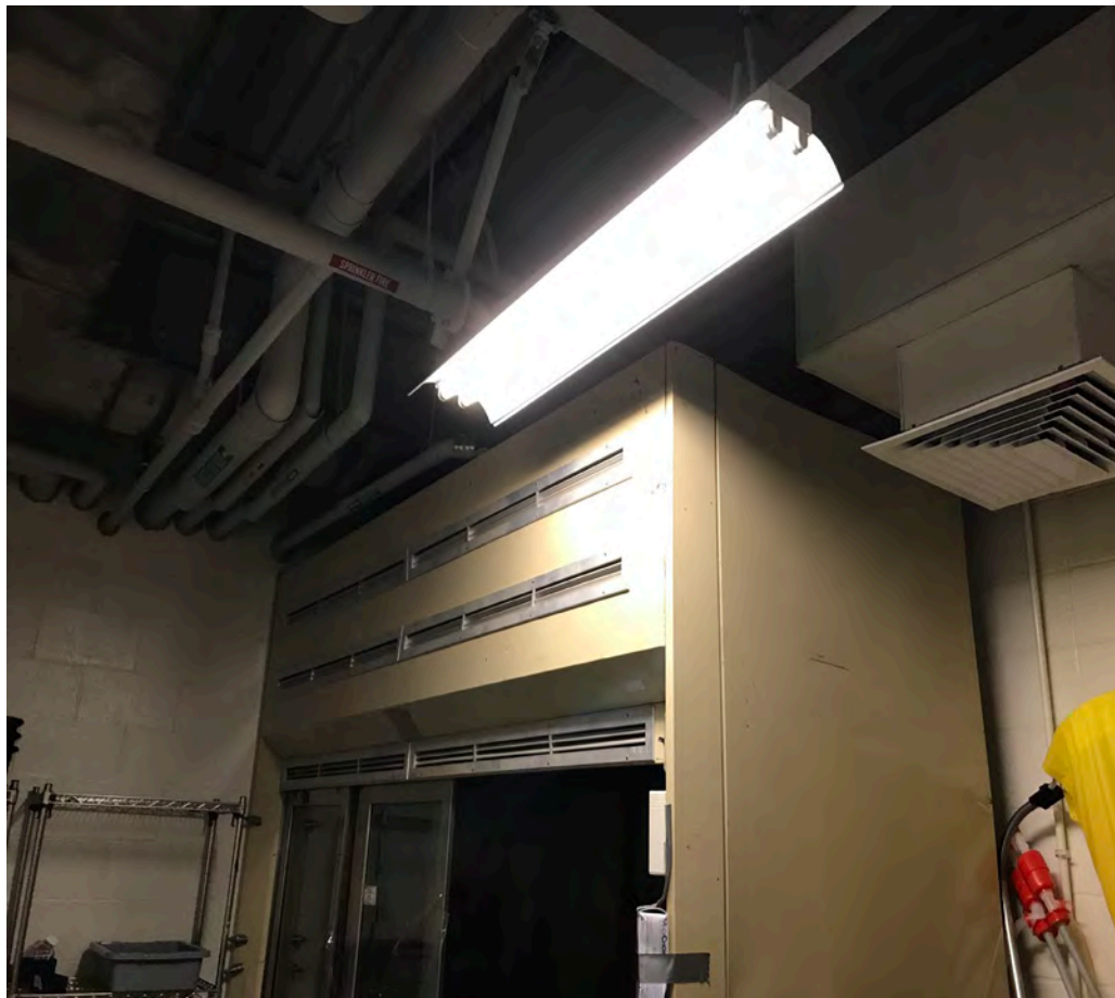
Photo 2 – Existing fume hood to be replaced
