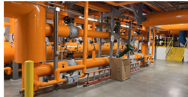
SUP Interior View of 125 psi Steam Header
