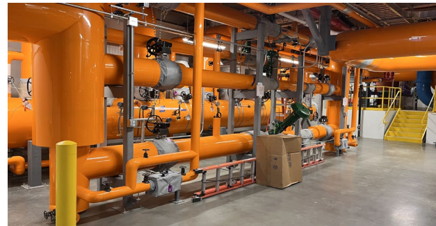
SUP Interior View of 125 psi Steam Header
