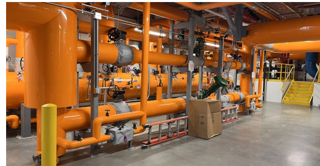
SUP Interior View of 125 psi Steam Header
