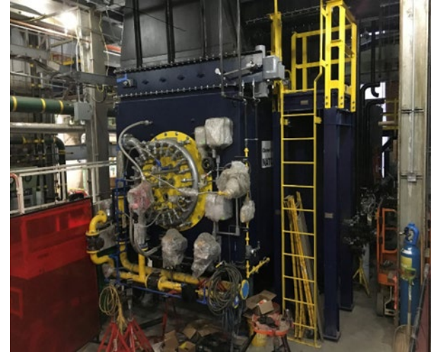
New Boiler installed in the Central Utility Plant
